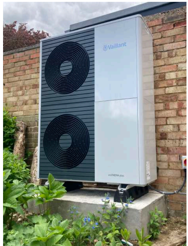
More homes are installing Air Source Heat Pumps and EV chargers for cars
